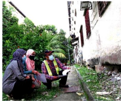
Taman Teluk Gedung Indah low-cost flats owners are hoping that their soil settlement issues will finally be resolved next year. – Filepic
